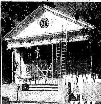
In a statement of national support, construction workers placed a Colonial 13-star flag on the Colonial-style building site where the Unitarian Church in Summit is making an addition.
