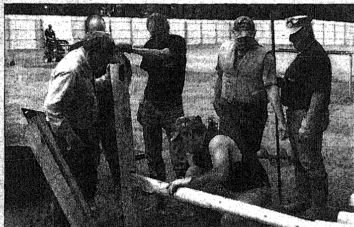
Setting the fence separating the observation area from the archers, Louis Sarmiento Jr. places the bottom rail into place as his father, Louis Sarmiento Sr., far left, looks on. Holding the post in place is George Anest, while Tony Bretones of Roselle and Ray Szpond Sr. wait before getting the next split rail ready.
