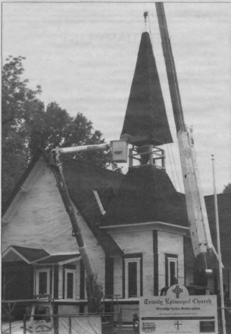
A new spire was installed at Trinity Episcopal Church at the corner of North and Forest avenues in Cranford.
