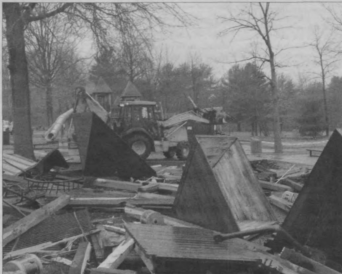
Union County work crews clear the old Loop playground in the heart of Union County's Watchung Reservation. The new playground is expected to be completed in the Spring, depending on the weather. The Watchung Reservation extends over five communities, Berkeley Heights, Mountainside, Springfield, and Scotch Plains, in Union County and Watchung in Somerset County.
