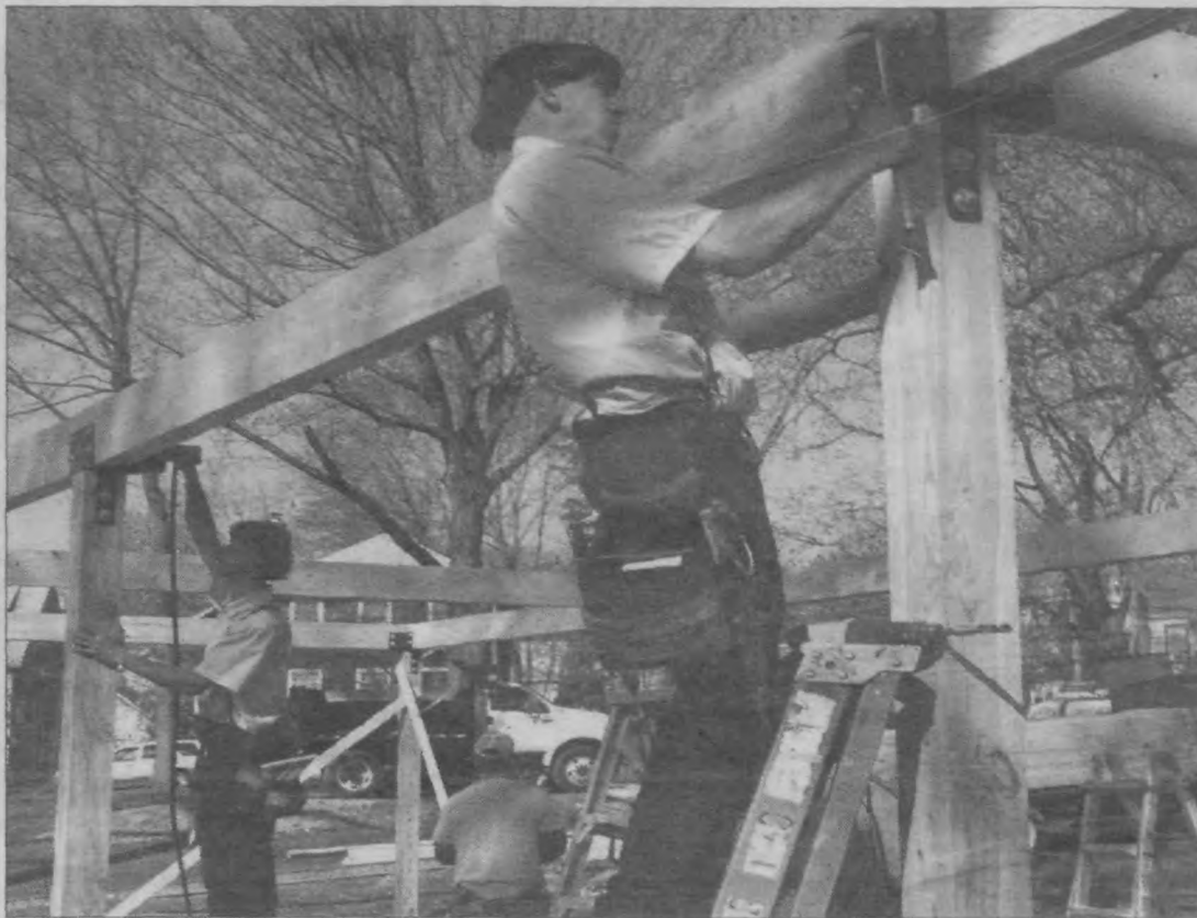
Leon Stoltzfus, right, and Samuel Stoltzfus of Lapp Structures secure the timbers of the Summit Bocce Pavilion. The long awaited Bocce Pavilion for the Summit Seniors Bocce Program arrived April 4. Within hours, a group of Amish builders had the structure erected to the delight of the Summit Senior Bocce Club.
